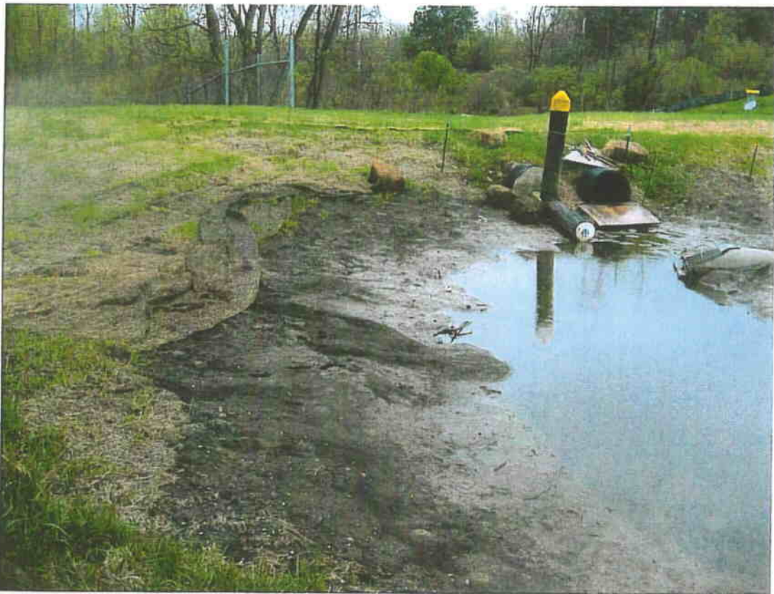
Figure 4-Re-pin erosion blanket in basin area, remove sediment from riser fabric, and seal opening of the north culvert so all storm water will flow thru the perforated riser.
