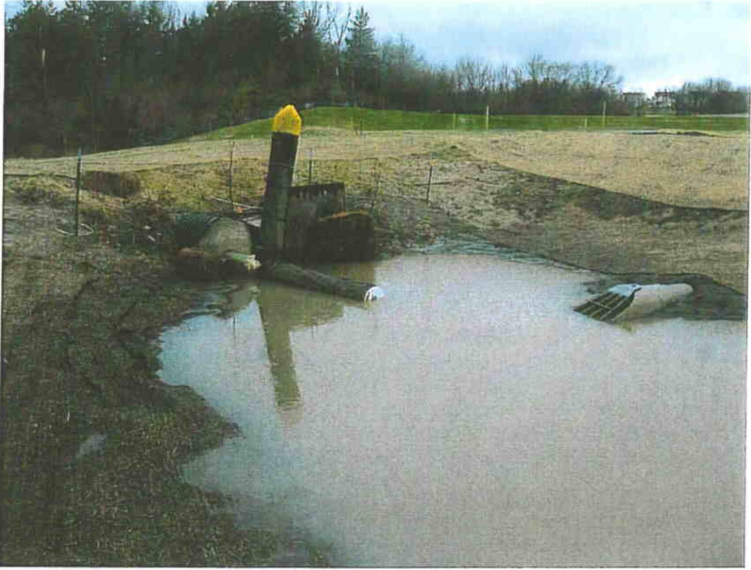
Figure 3-Perforated riser has been re-set to vertical position in basin.
